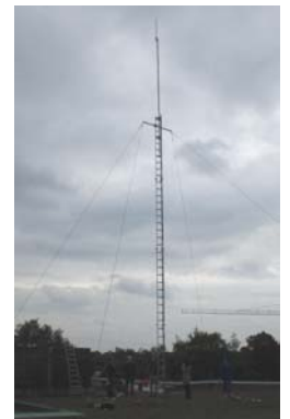
New tower and antenna
